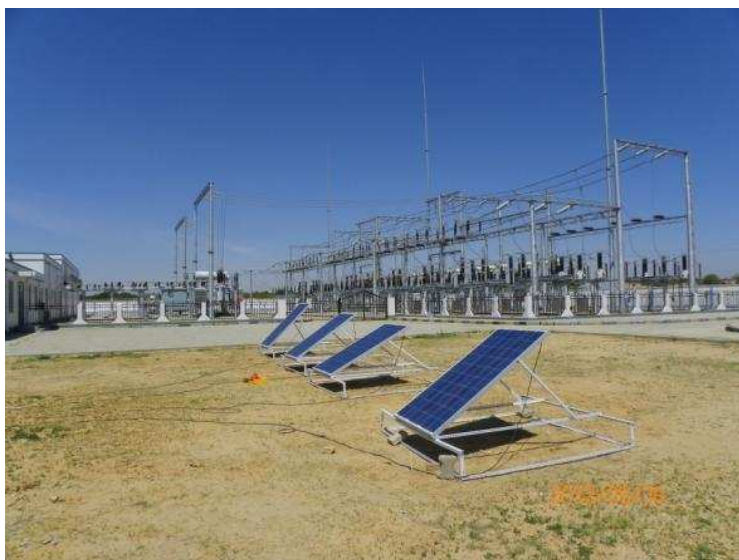
Figure 3. Solar module in the 110kv substation of Yulin Mazhaliang
